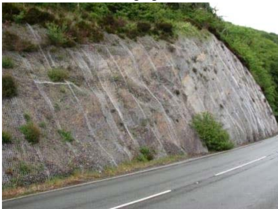
Fig. 5: Gabion wire mesh used to prevent rock fall from highway slopes
