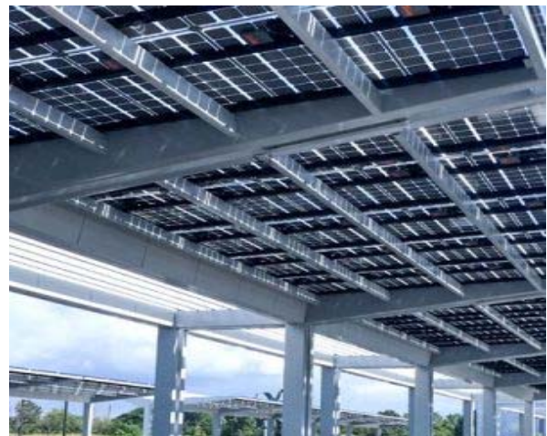
Figure BIPV System as Roofs
